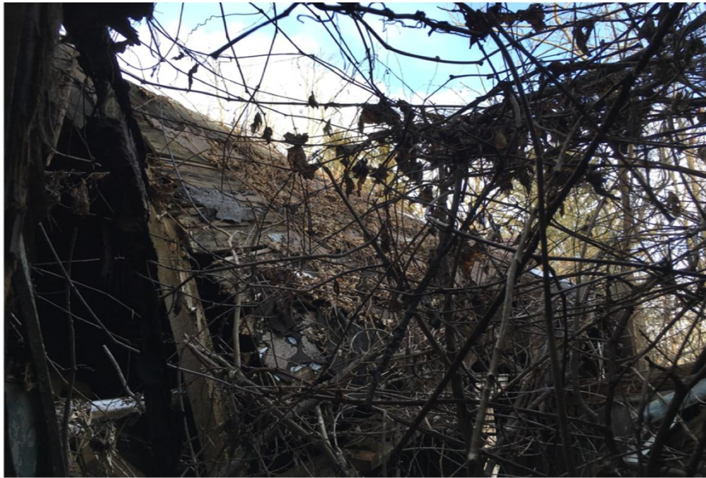
PHOTO VIEW: 4 - Collapsed Structure - Potting Shed and Summer Kitchen
